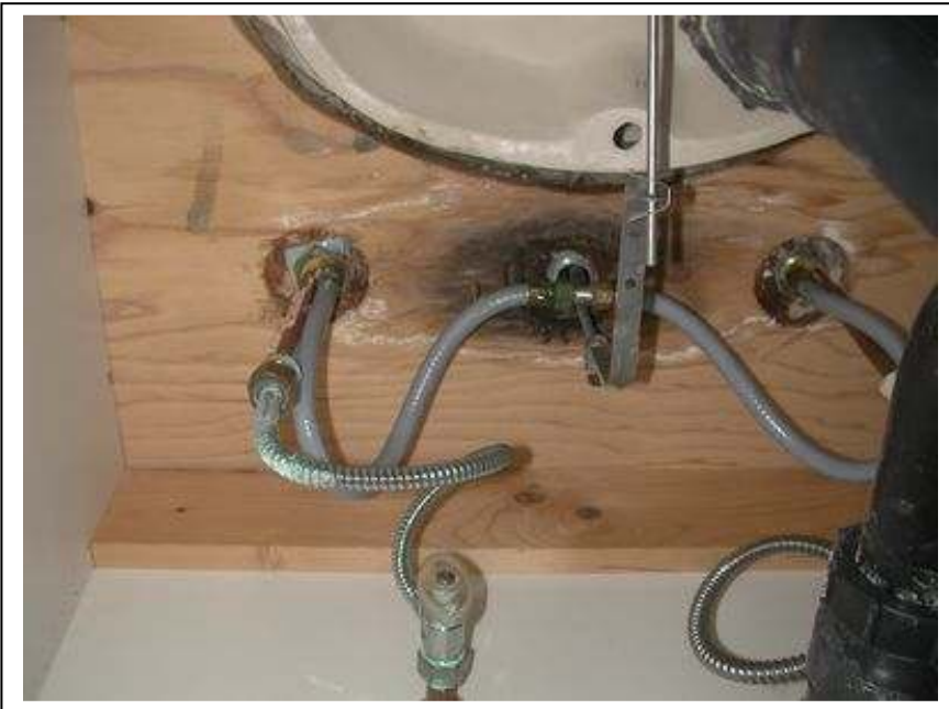
019. CR.H.2373. The right sink in the master bath had a leak around the spout and that water has damaged the wood sub cabinet and dripped on the base of the cabinet damaging the base.
