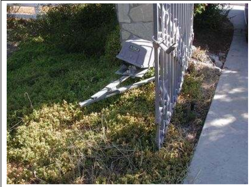
Figure 001. CR.H.2252. There are electrically operated gates at the driveway entrance that are in disrepair and do not move and the remote control for them was not found.
