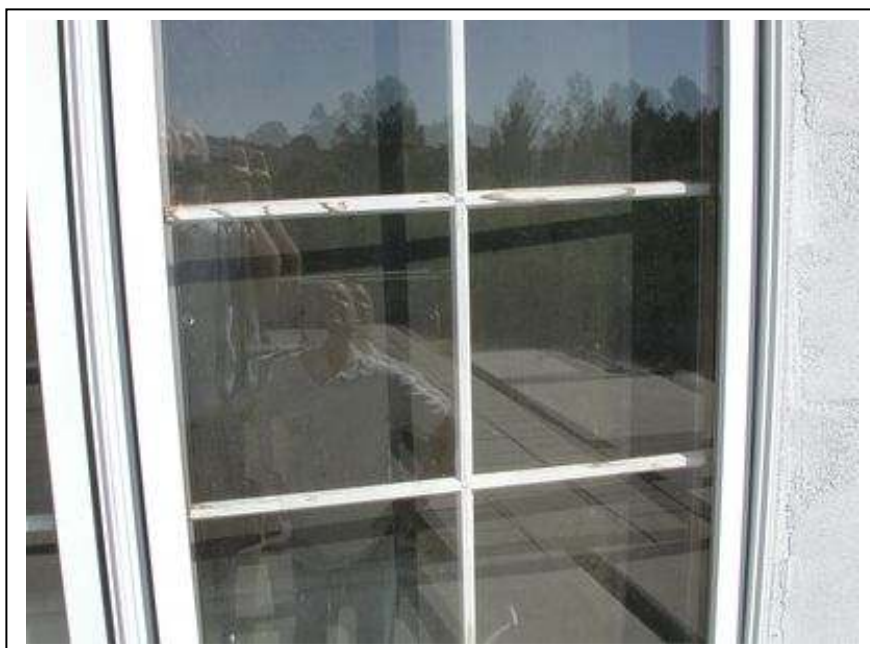
14. CR.PTR.2273. There are many windows with grids that are deteriorating from weather.
