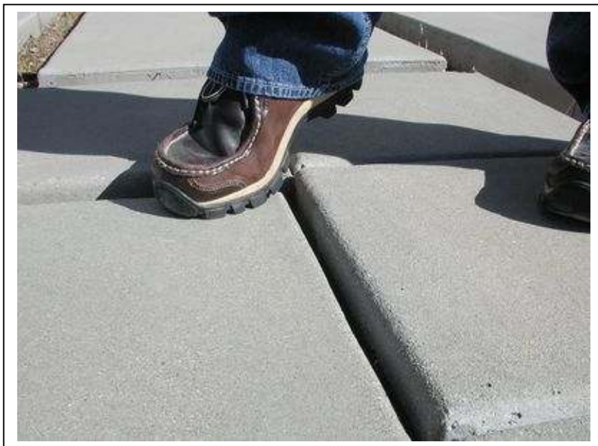
017. CR.H.2278. The decking has some concrete pieces that are loose.
