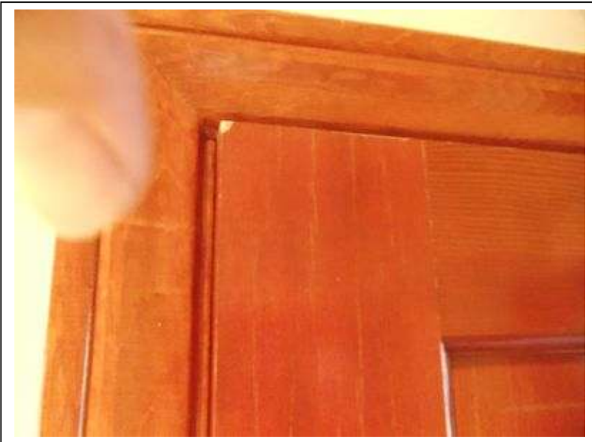
003. CR.H.2439. Bathroom door in secondary restroom is sticking, requires adjustment
