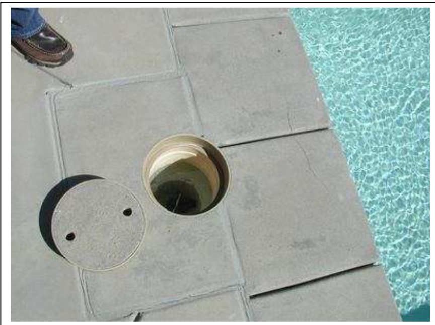
004. FE.C.2340. The pool perimeter deck is of concrete and there are no cracks in it except right at the skimmer at the shallow end, recommend review by pool contractor.
