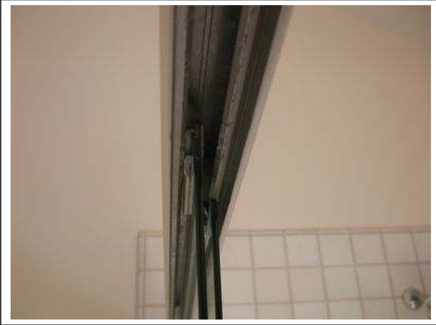
018. CR.H.2372. The sliding glass doors at the master bathroom shower are not suspended properly.
