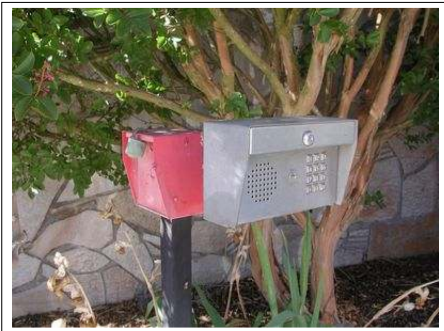
002. FE.C.2253. There is an intercom at the front entrance that could not be tested and there is a red box with a key that is likely for the fire department and should be investigated further.
