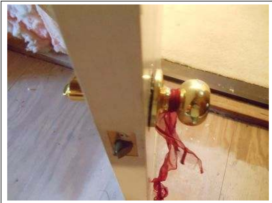
Figure 001. CR.H.2437. Door handle loose at attic above garage
