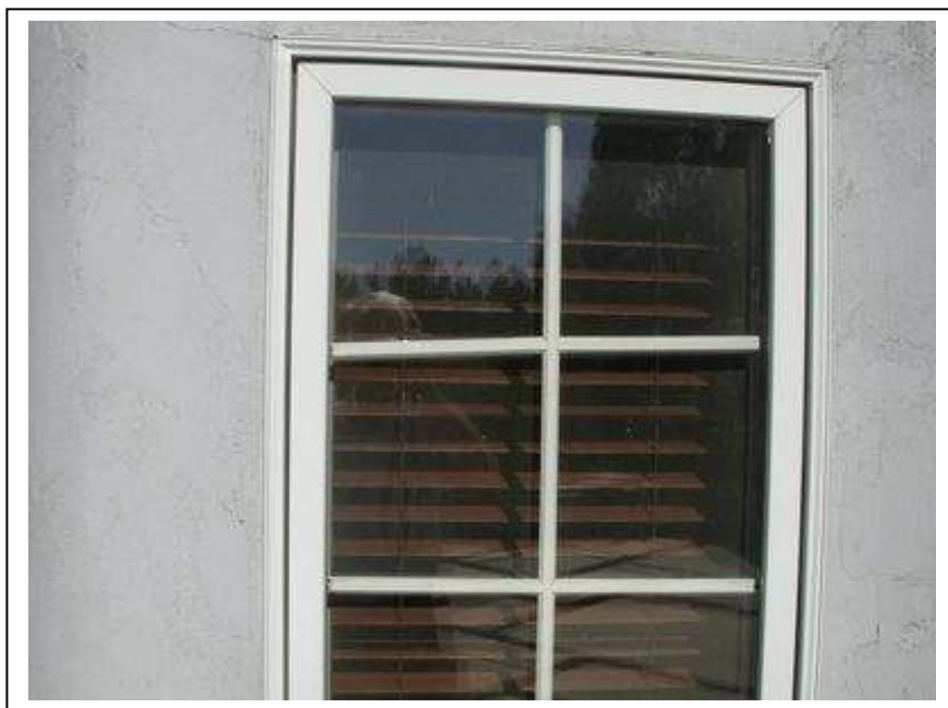
13. CR.H.2272. There are some windows that have grids that are sagging.
